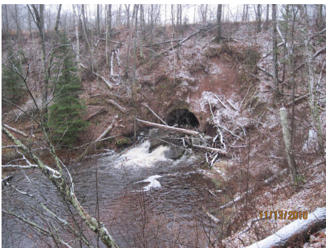
Nebagamon Ck as it flows thru collapsing culvert under the South Shore Railroad Grade
